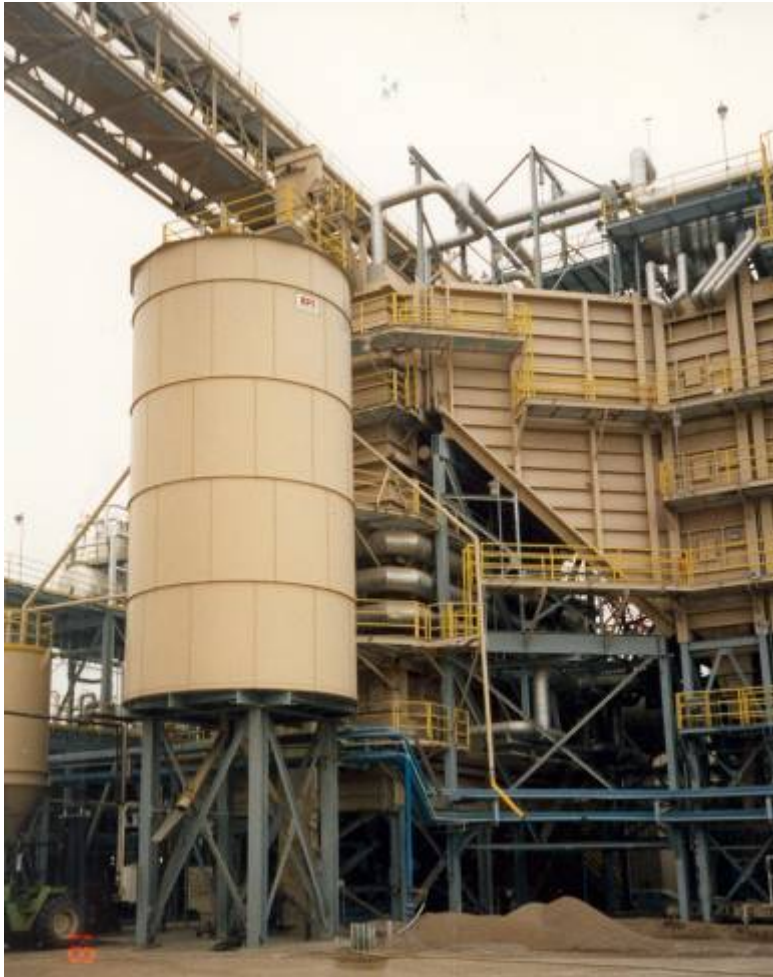
Feed Conveyor Lime Silo and Fluidized Bed
